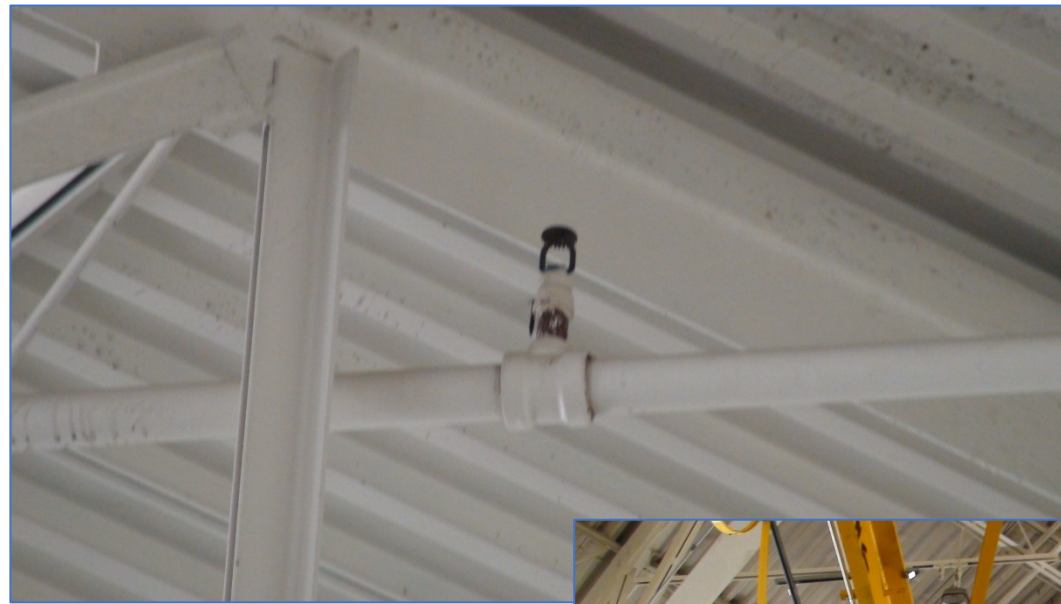
Photo 3: Water-based deluge system sprinkler, facing south
