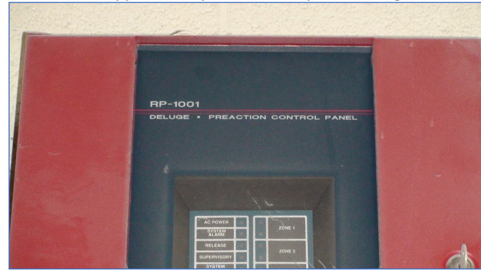
Photo 2: Fire suppression system control panel, facing south
