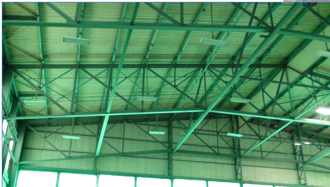
Photo 4: Hangar area fire suppression deluge sprinkler system
