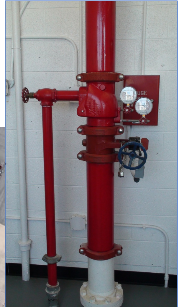
Photo 3: Wet-pipe fire suppression system valve, facing west
