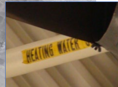
Photo 5: Hydronic heating system pipe
