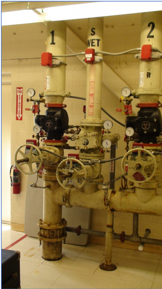
Photo 1: Fire suppression deluge valve system, facing west
