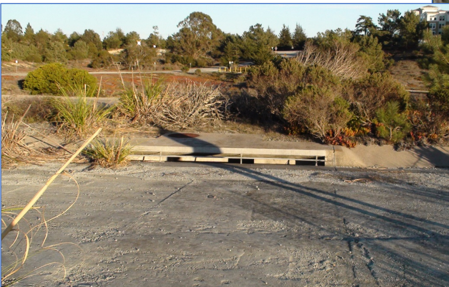
Photo 3: Stormwater drain inlet (discharges to drainage ditch on 5 th Avenue), facing east
