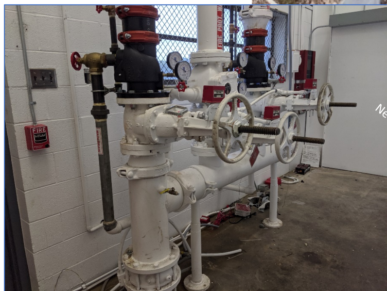
Photo 4: Fire suppression system deluge valves, facing northwest
