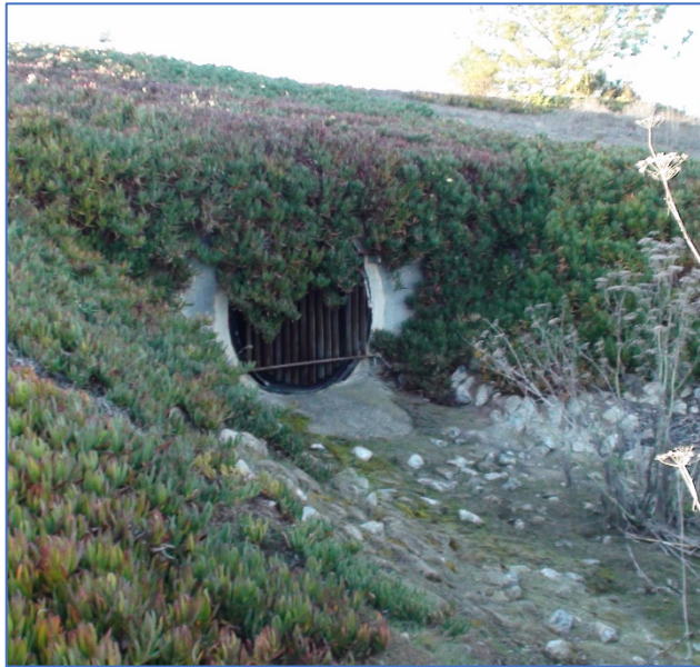
Photo 5: Stormwater outlet from Site 17 to Pete's Pond, facing northwest
