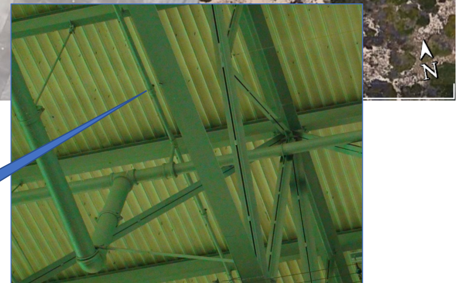
Photo 3: Hangar area fire suppression deluge sprinkler system
