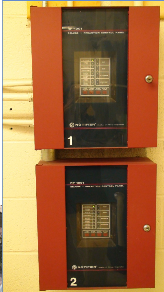
Photo 2: Fire suppression system control panels, facing west
