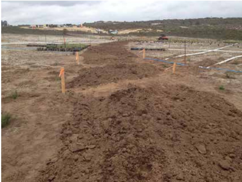
Photograph 23 – Interim Action Ranges MRA Range 47 Restoration Area. Temporary restoration area road after soil ‘ripping,’ looking east. 5 February 2013
