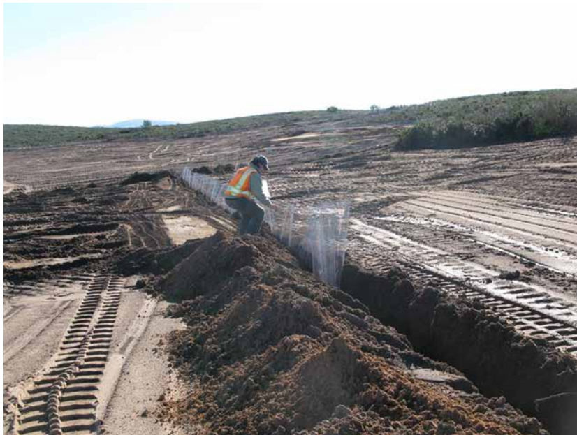
Photograph 8 – Interim Action Ranges MRA Range 47 Restoration Area. Below-ground fence installation to exclude burrowing animals. 7 January 2013
