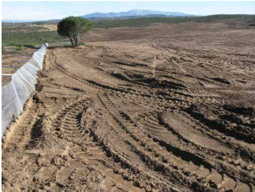
Photograph 9 – Interim Action Ranges MRA Range 47 Restoration Area. Restoration area during fence installation, looking east. 7 January 2013
