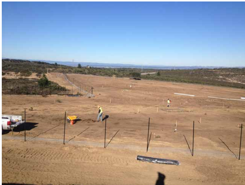
Photograph 10 – Interim Action Ranges MRA Range 47 Restoration Area. Fence installation, looking north. 14 January 2013
