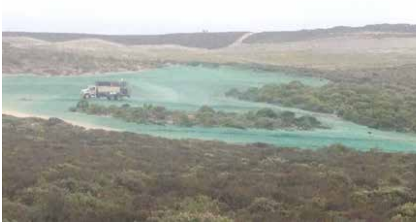
Photograph 29 – Interim Action Ranges MRA Development Parcel. Hydromulching for control of wind erosion, looking south-southwest. 11 July 2013
