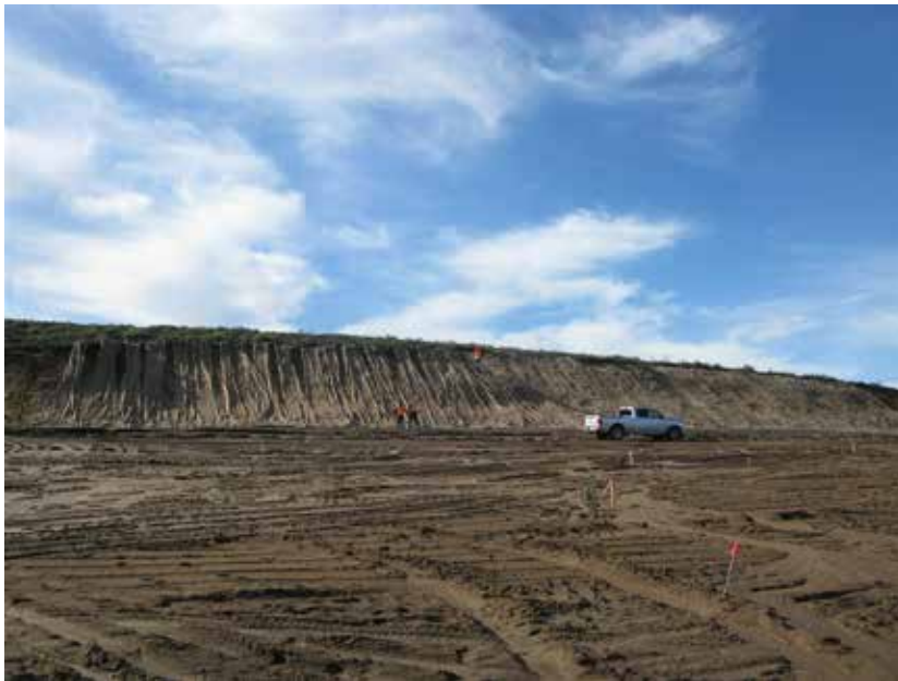
Photograph 12 – Interim Action Ranges MRA Range 47 Restoration Area. Erosion control blanket installation on escarpment. 7 January 2013
