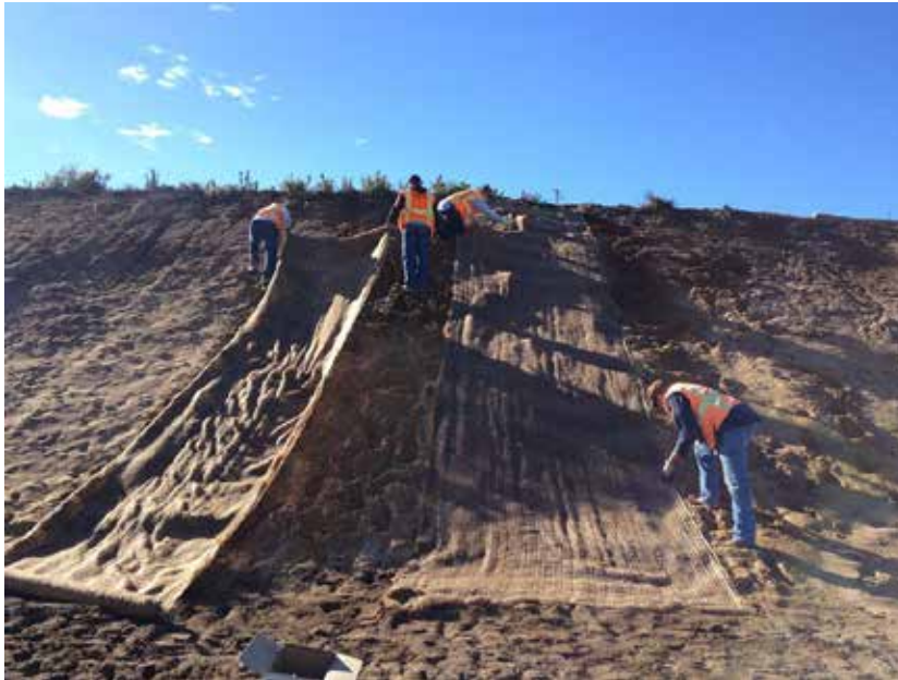
Photograph 11 – Interim Action Ranges MRA Range 47 Restoration Area. Erosion control blanket installation on escarpment. 3 January 2013
