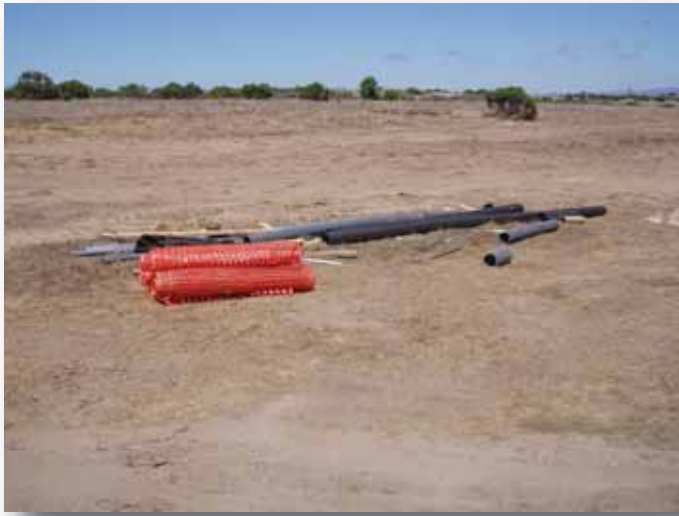
Photo 9. Piping at site 3 uncapped (looking Northeast).
