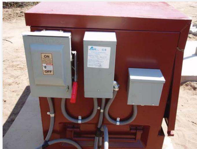
Photo 22. Transformers mounted on metal well cover at well MW-OU1-46-AD.
