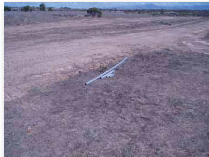
Photo 28. Piping left in staging area. Caps missing on pipe ends (looking Northeast).
