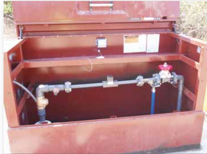
Photo 26. Well pump inside of metal box at well MW-OU1-87-A.
