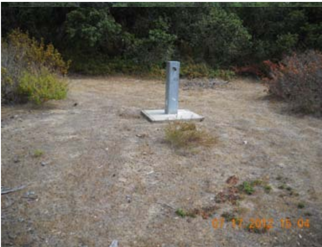
WCS# 10B ps30a MW-OU1-59-A Post-Treatment 17 July 2012
