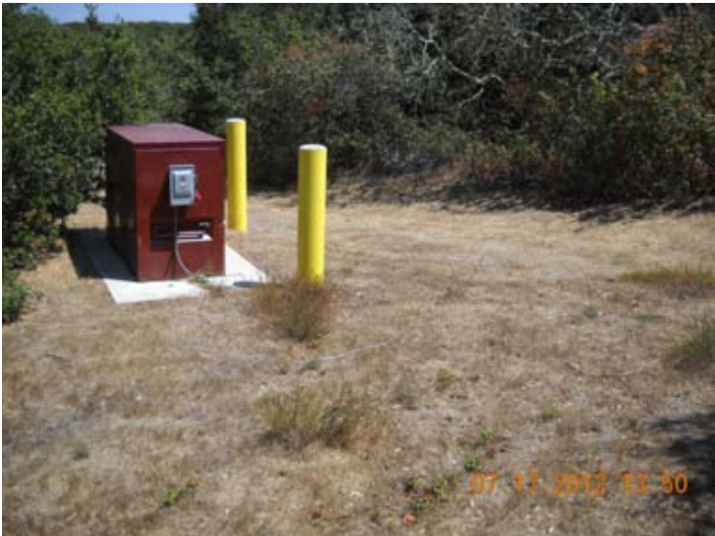
WCS# 12B ps48a MW-OU1-85-A Post-Treatment 17 July 2012
