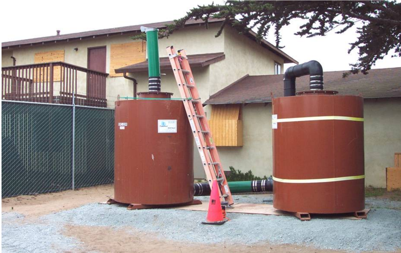
Photograph 2-6 Granulated Activated Carbon Units
