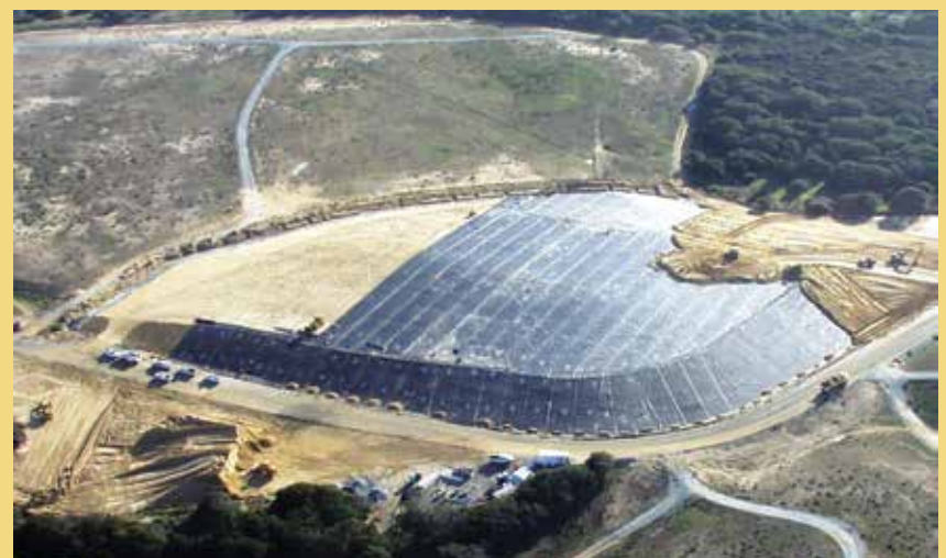
Landfill during installation of the engineered cap and covering with natural habitat
