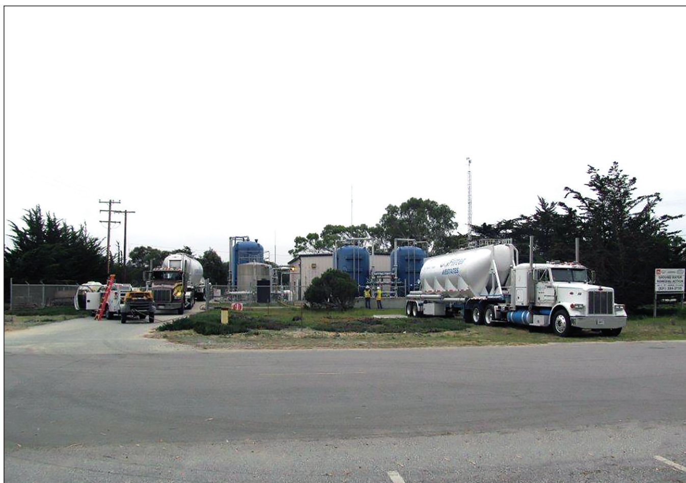
Operable Unit 2. The existing granulated activated carbon (GAC) is changed-out with fresh granulated activated carbon. The GAC is in the large blue tanks.
