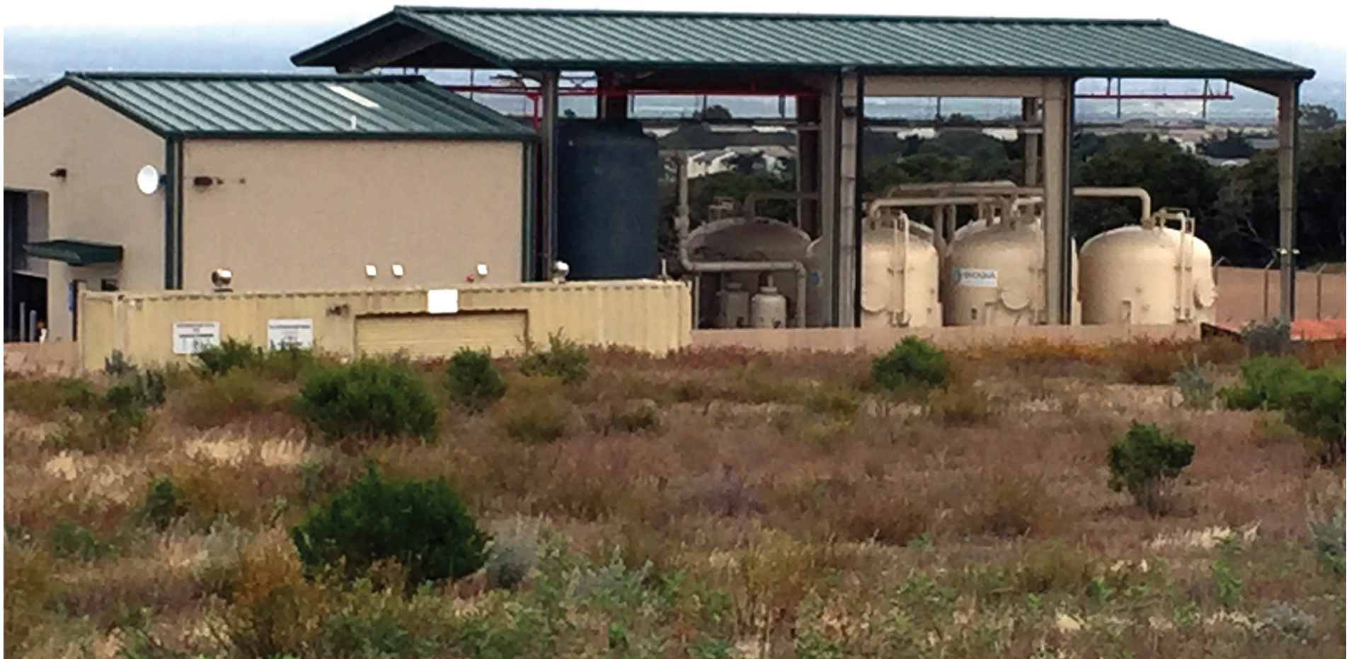
New Operable Unit 2 Groundwater Treatment Plant located within the landfill property.
