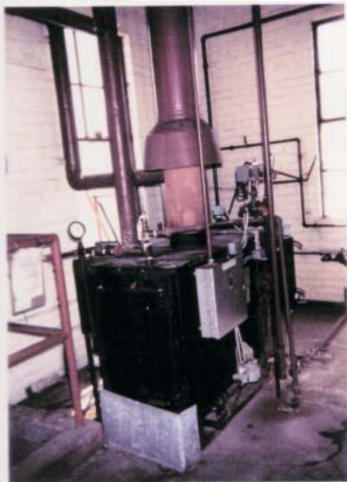
Site 17, FTO-013, Building 1442 Autoclave
