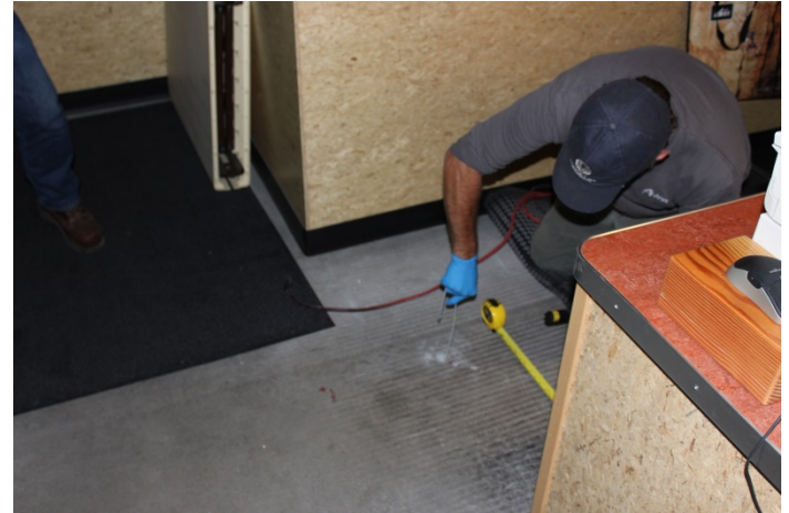
Picture 2. Installing soil gas probe SG-12-27 in the REI southwest checkout area
