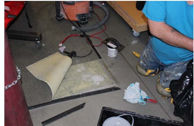
Picture 4. Sub-slab borehole patched for soil gas probe SG-12-28 in the REI center retail area
