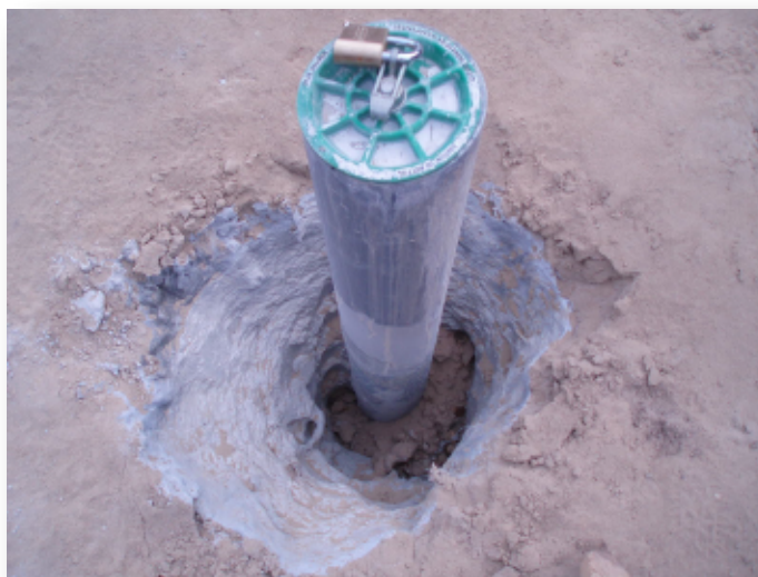
Photo 39. EW-OU1-71-A representative of wells surrounded by a depression after settling of concrete. All depressions were subsequently filled by HGL field staff.
