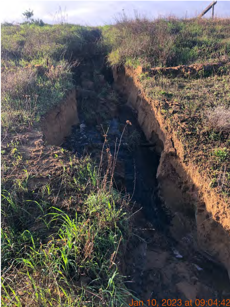
Area F vegetative cover erosion damage
